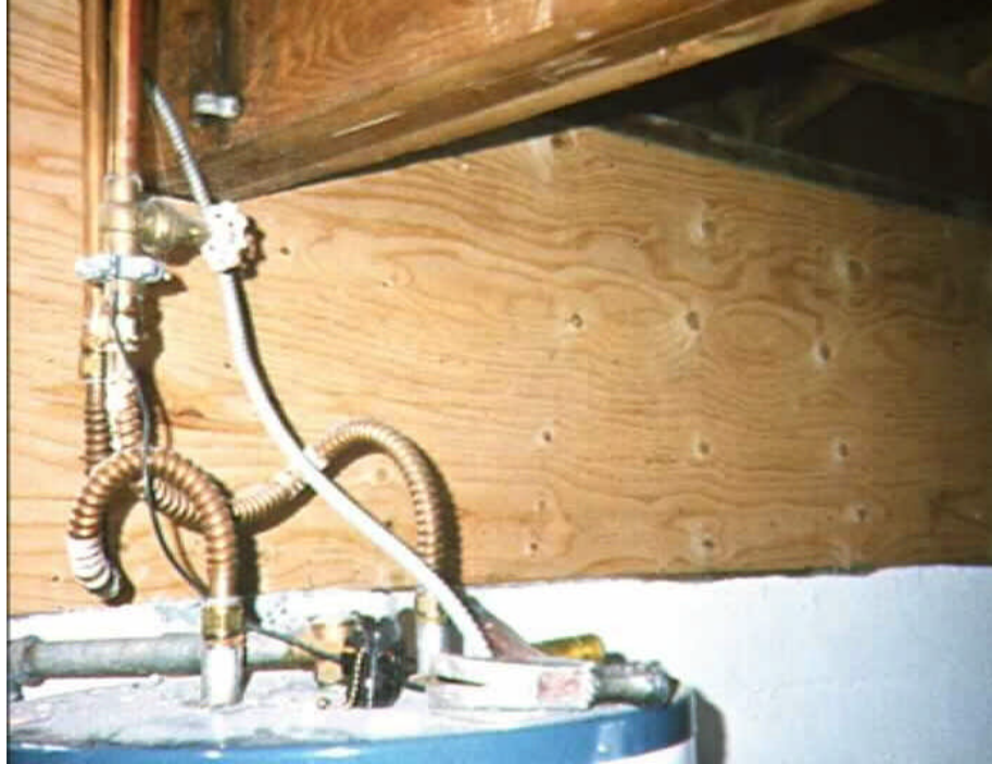
Figure 10 Refer to the Plan Detail Reference sheet (Plan Detail 2d) to determine how to cut-out a section of the structural panel to accommodate piping, etc. (Photo from Ben Emam, Amazon.com)
