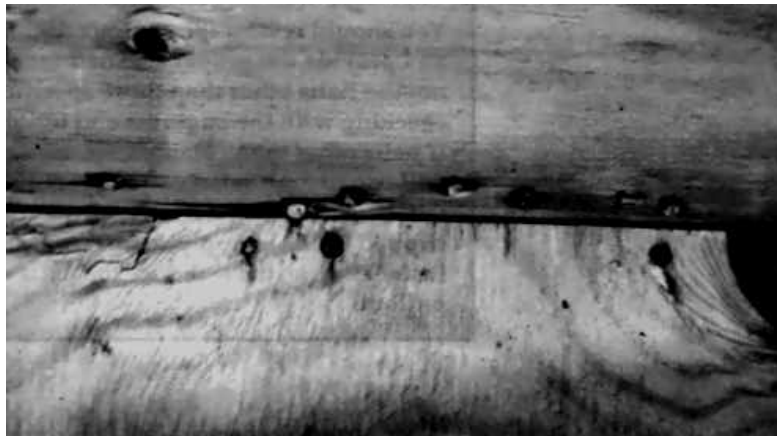
Figure 12 An example of overdriven nails and nails too close to the panel edge. Nails should be driven flush with the surface of the structural panel.
