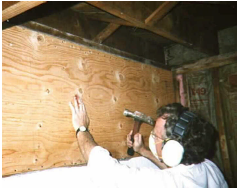
Figure 9 A structural panel installed to strengthen the pony wall to prevent the wall from collapsing, causing the home to fall off the foundation. (photo from Ben Emam, Amazon.com)
