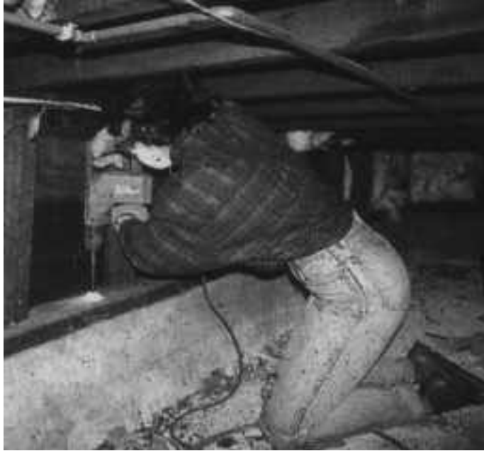
Figure 4 Installing anchor bolts into the sill plate using a rotohammer. Note that the sill plate is wider than the pony wall studs. (Photo from City of San Leandro)
